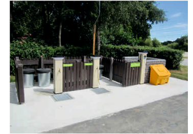
Low level lights at water point
