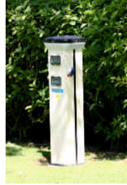
Low level light at electrical hook-up
